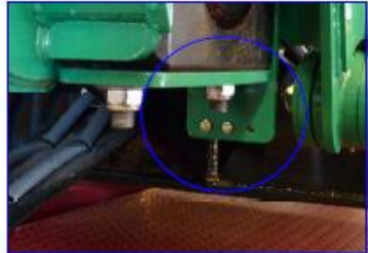
GREASE BLOCK FOR PINS & BUSHES 5 POINTS FRONT 5 POINTS REAR
